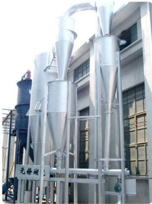
Gasifier - dedusting system
