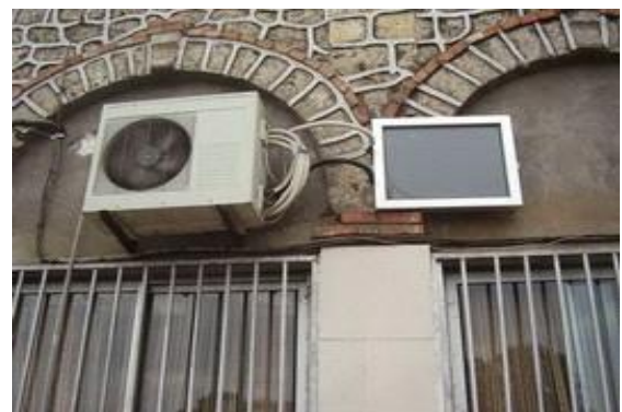
Our Solar AC used in Africa office
