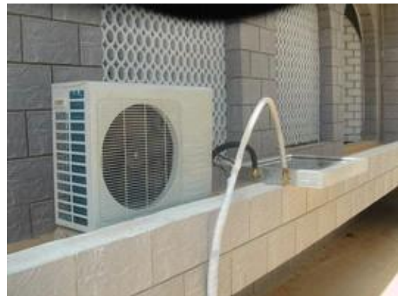
Our Solar AC used in Sharjah building
