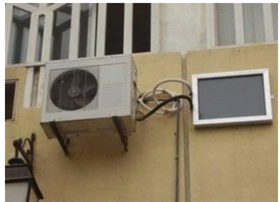
Our Solar AC used in Africa building
