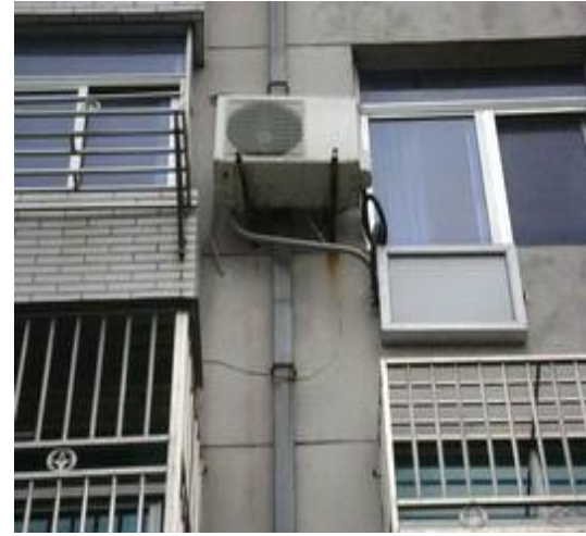
Our Solar AC used at home
