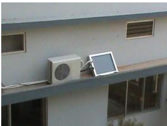
Our Solar AC used in Africa building
