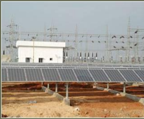
6.Solar Power Plant(Turnkey)
