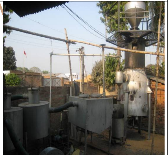
Rice husk Based system for paper making unit in operation for 14 months – duel fuel mode
