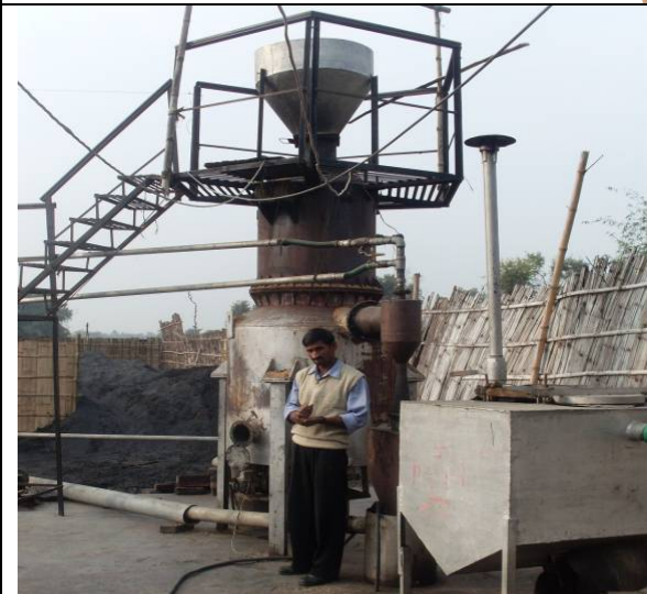
Rice husk based 100 % producer gas System in operation for last 18 months covered over 7500 hours of operation without any failure
